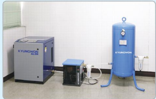
▶ Installed in spacious space
