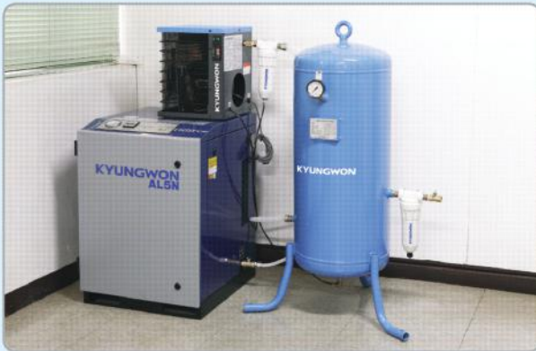
▶ Installed in narrow space
